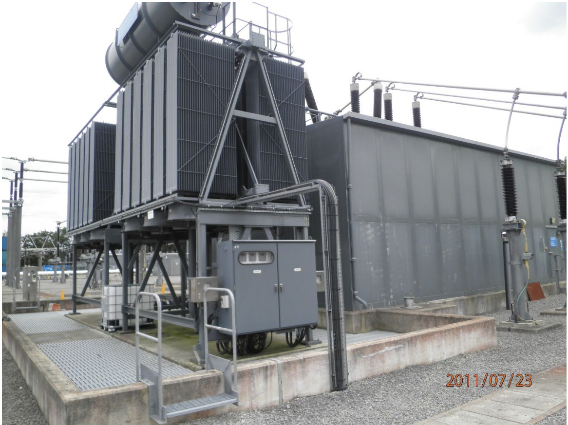
Plate 4.9 Typical (large 400kV) power transformer
